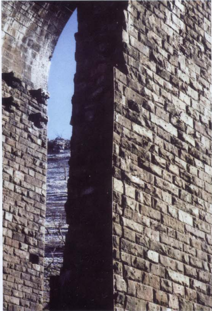
Cracked and damaged piers, Smardale Gill Viaduct, 1990. Photo: Gordon Biddle
